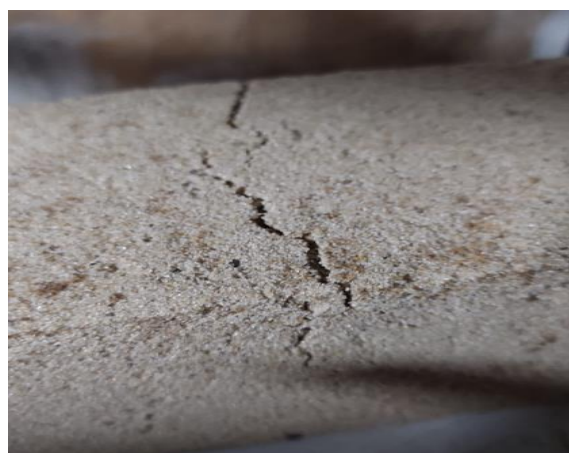
Figure 18 Zoom on Beam on failure. 30% of SS21
