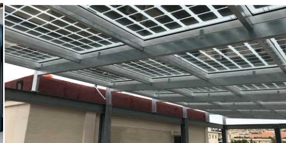
Fig.15. PV canopy of Private House in Nablus
