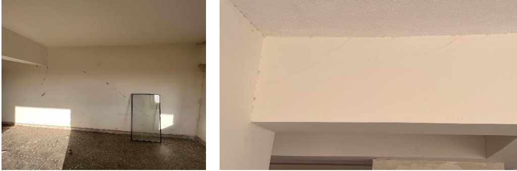
Fig 13: Other elements condition in same building:
