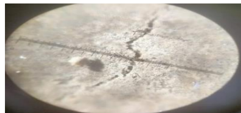
Figure 21- Crack pattern of slab C6
