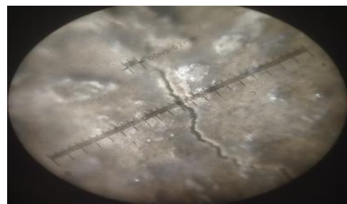
Figure 20- Crack pattern of slab C5
