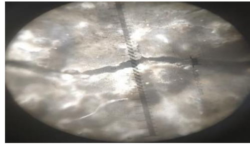
Figure 17- Crack pattern of slab C2
