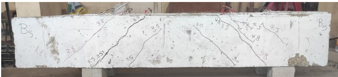
Fig. 14. Crack patterns at failure of specimen (B5).
