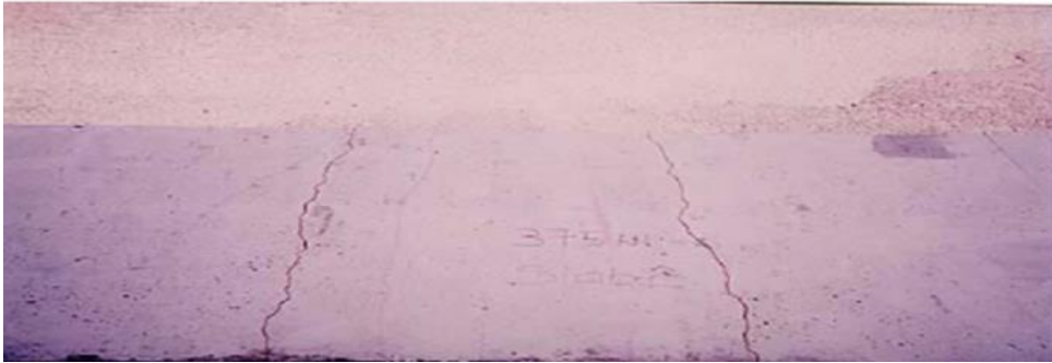
Fig. 4: Crack shape before reservation [18]
