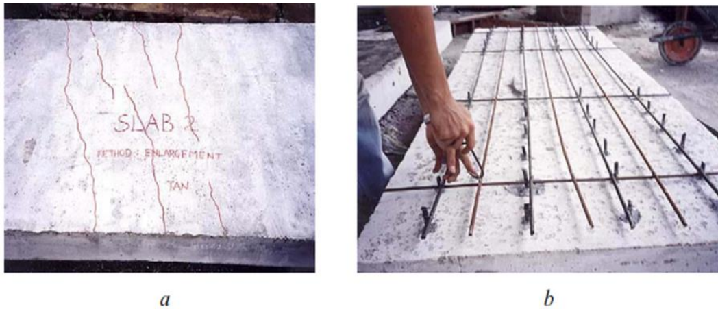
Fig. 7: Strengthening by increasing the area of the slab: (a) cracked pattern prior to restoration; (b) a surface that has been roughened and steel supplied [18]
