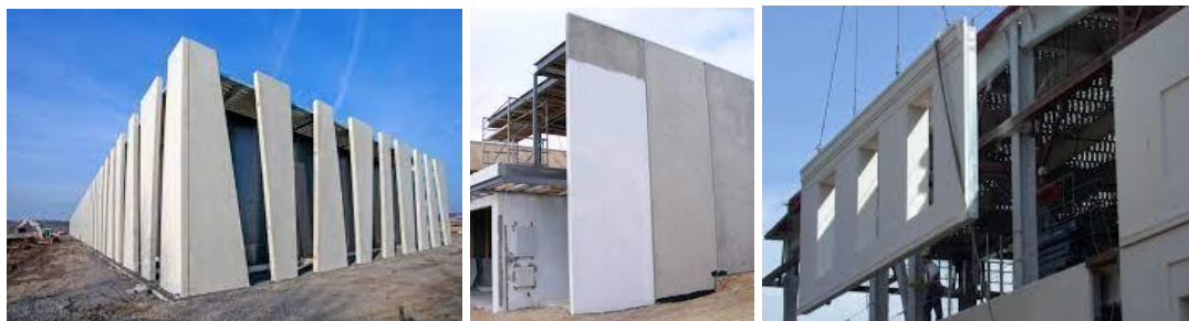
Fig. 17. shows some tybs of pre cast concrete before pouring into the facades
