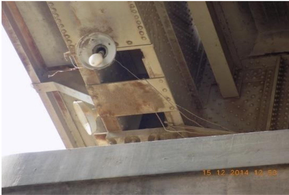
Fig.(23) Poor Lighting System, Marazek Bridge
