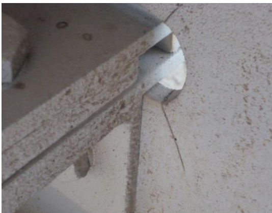
Fig.(6) Fatigue Crack at Stringer-to-Cross Girder Connection, Abo Shosha Bridge
