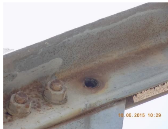
Fig.(12) Missing rivet – Edfina bridge
