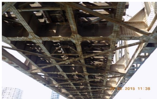
Fig.(4) Corrosion and rusted floor members – Banha Bridge
