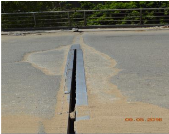
Fig. (10) Poor Condition of Expansion Joint, Sanae Bridge
