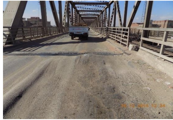
Fig.(20) Settlement of Wearing Surface, Marazek Bridge
