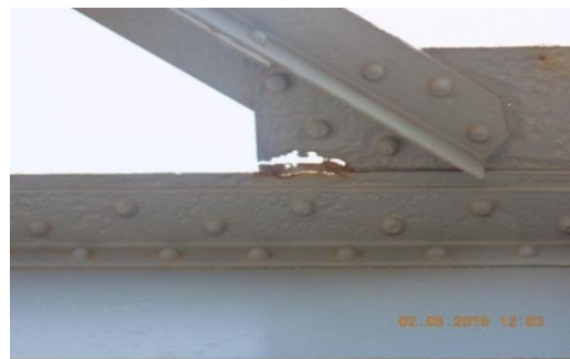
Fig.(5) Corroded plate due to severe oxidization – Kafr El Zayat Bridge
