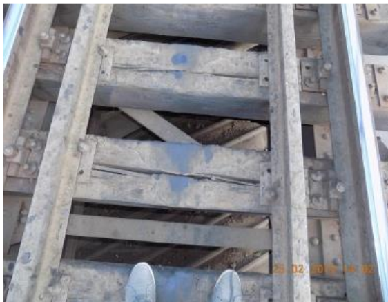
Fig.(21) Condition of Sleepers, Banha Bridge Rail and slipper defssionses
