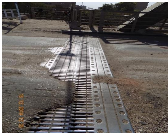
Fig. (8) Creep of Asphalt over the Expansion Joint, Marazek Bridge
