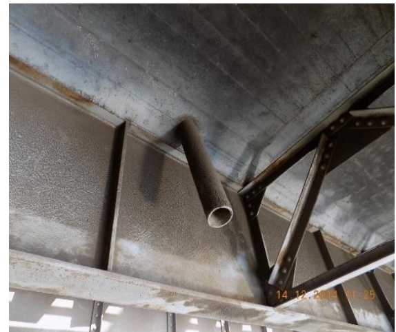
Fig.(22) Improper Drainage System, Marazek Bridge
