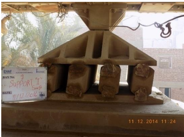
Fig.(17) Distortion of Roller Bearing due to Abutment Movement
