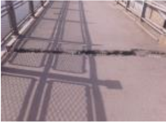
Fig.(19) Cracking of Concrete, Imbaba Bridge
