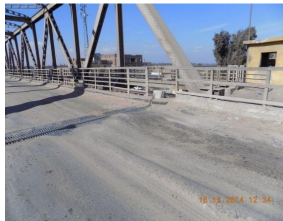
Fig. (9) Settlement of Approach Slab at Entrance of Roadway Lane, Marazek Bridge
