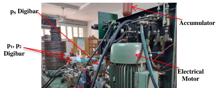
Fig. 5 Photograph of the rear view of hydraulic control system.
