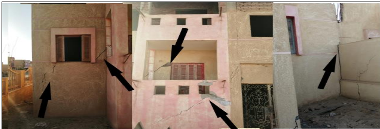
Fig. (10): Borehole (B.H.20) was drilled near the defected building.
