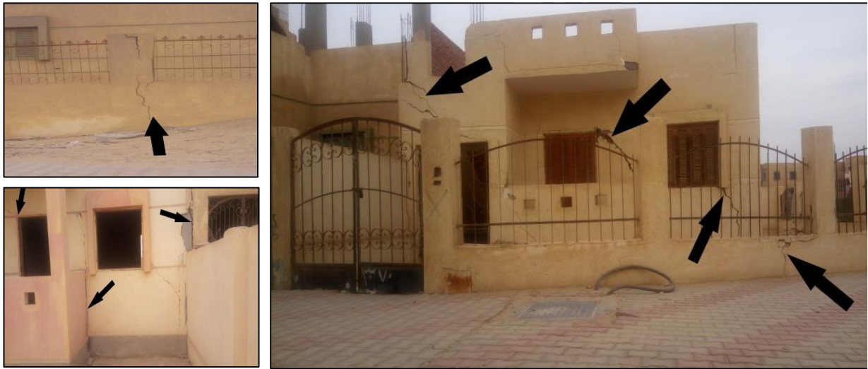
Fig. (12): Cracks observed at light structures.
