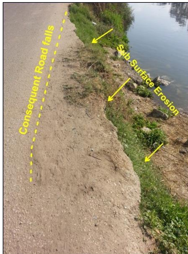
Fig. (4): The southwestern shoulder of the submerged Siphon body.
