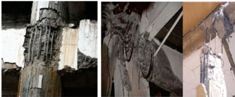
Fig. 1: Beam–Column Joint Failure.
