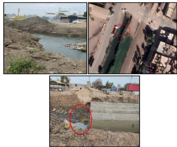
Fig. 11. Contracted cross-section upstream covered structure causing local scour.
