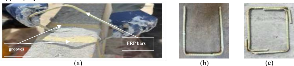
Figure 13. (a) Near-surface mounted NSM GFRP bar installation, (b) U- shape GFRP bar, (c)rectangular shape GFRP bar.[13]
