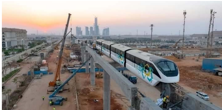
Fig. 4. Implementation of the New Administrative Capital Monorail source: National Authority for Tunnels, 2023 (Projects, 2020)
