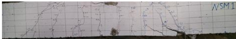
a) Crack pattern and mode of failure for beam (NSM1).
