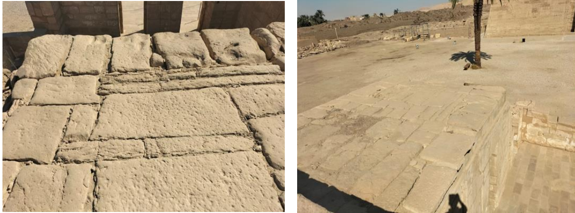
Figure 2a, b shows deterioration of Surface layer of stones on the roofs of Madinat Habu
