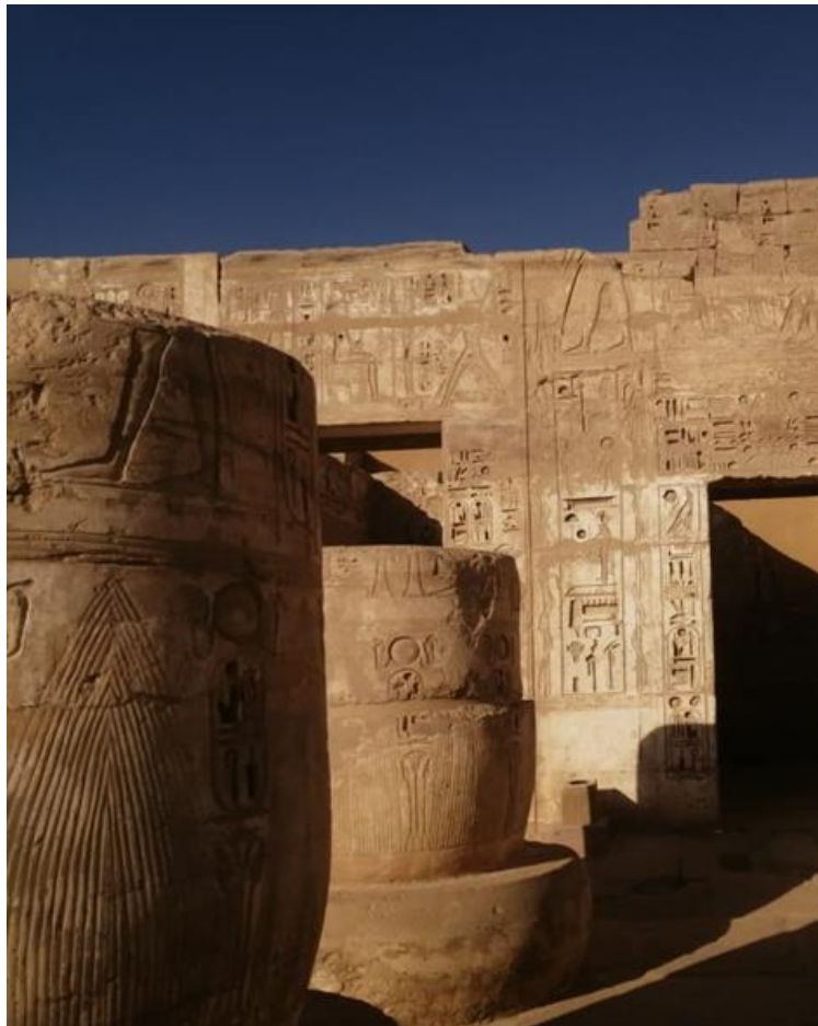
Figure 1. shows deterioration of the edges of the building stones on the roofs of Madinat Habu
