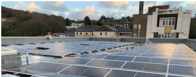
Figure 4: Applications of photovoltaic systems (stations installed on building rooftops) - [23]
