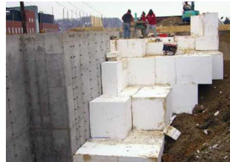
Fig 12 Geofoam retaining wall backfill for West Virginia, University student housing project, USA.
