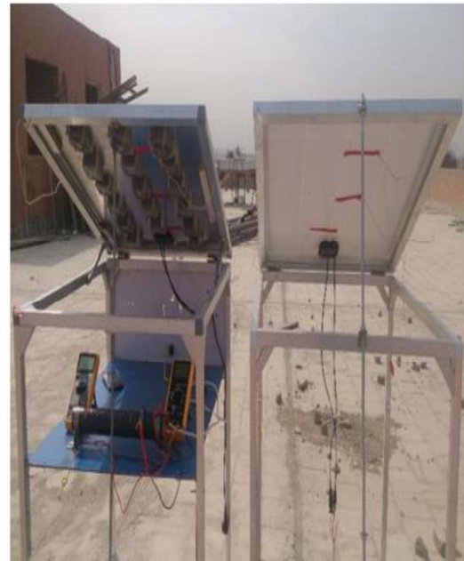
Fig 2: Back face of a PV modules with thermocouples.
