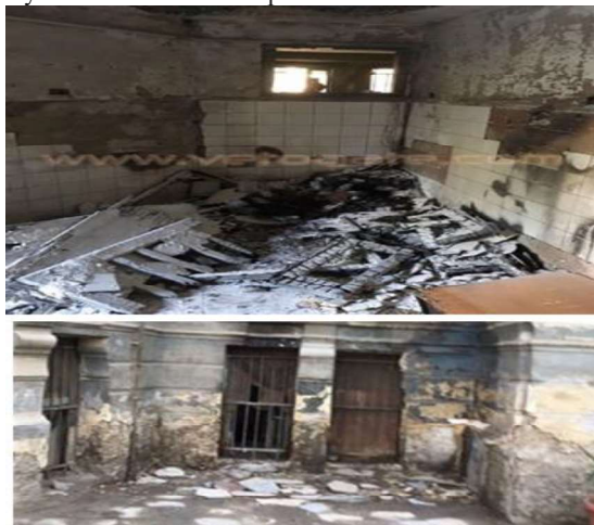
fig. 17&18: Pictures show the deterioration and damages in the Sakakini Palace as a result of not being properly and successfully re-used
