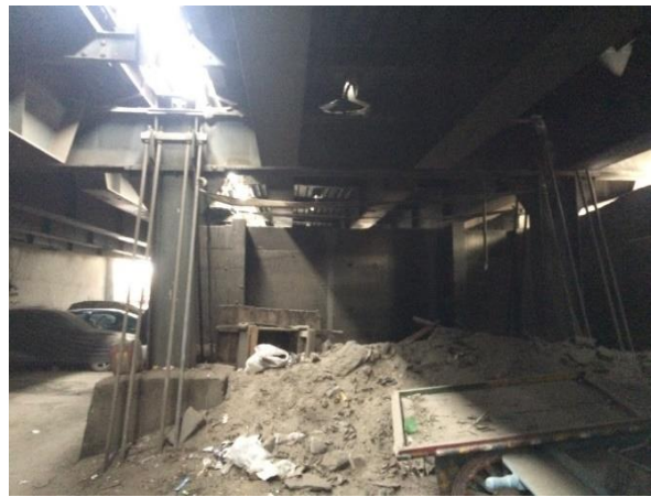
Figure 10: Accumulation Of Garbage Around Supporting Elements
