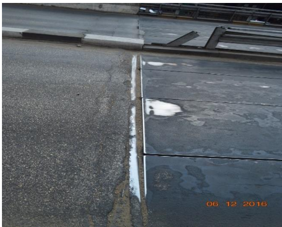
Figure 9: Loss Of Asphaltic Layer And Exposure Of Metallic Deck
