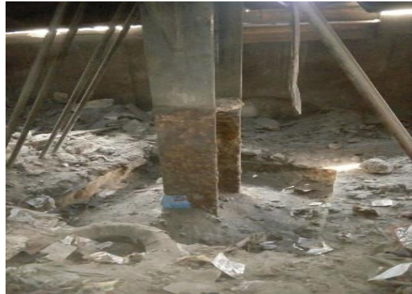
Figure 8: Corrosion At Bottom Of Bridge Columns
