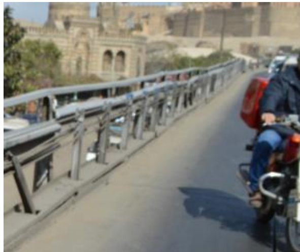
Figure 12: Bad Condition Of Guardrail
