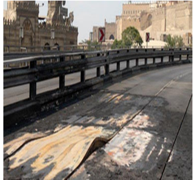
Figure 6: Permanent Deformations In Bridge Deck
