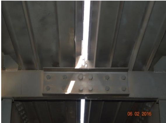
Figure 7: Loss Of Expansion Joints And Large Observed Distance Between Deck Parts
