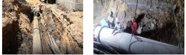
Figure 1: Actual case infrastructure damage.
