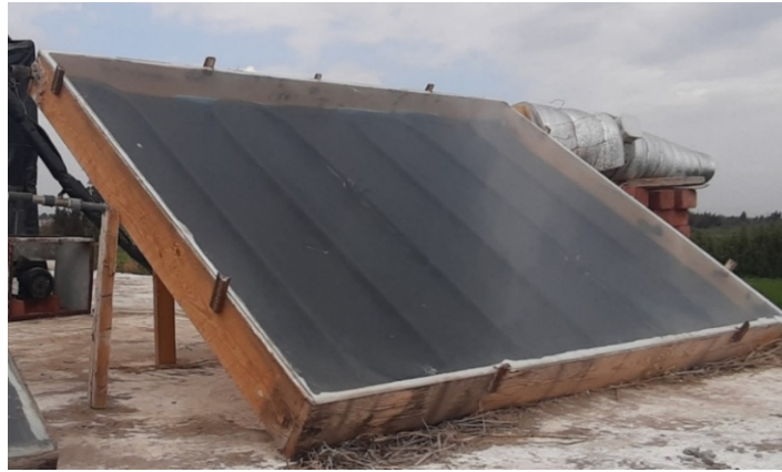
Figure (4): Solar air heater
