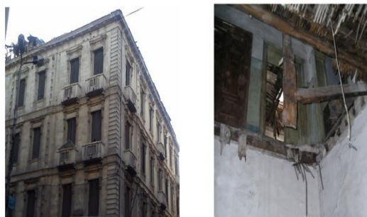
Figure 1 Ruined old building - a- Elevation of the building - b- the destroyed floor of old building
