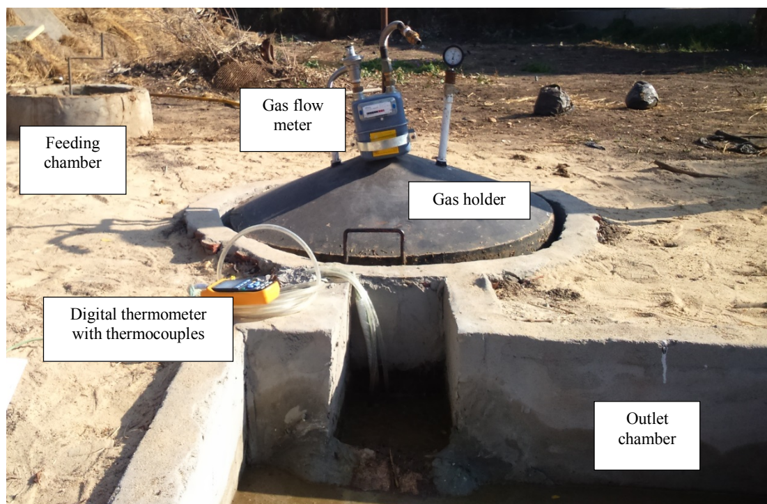
Fig.1. A view of the investigated biogas unit
