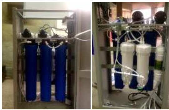
Fig 4: Photo of RO system
