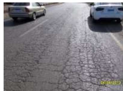
Figure 1. Excessive Alligator Fatigue Cracking (New Damitta- to Damitta Port Road)
