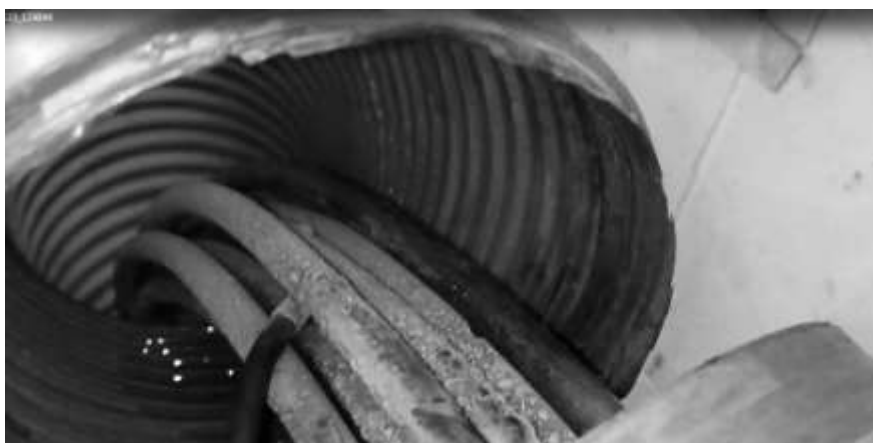
Figure (9): Frost formation on the inner tubes of the water cooler at no load test
