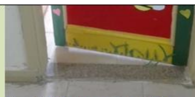
Fig. 28: Field photo of threshold loves the classroom door for disabled children; this impedes the movement of the child wheelchair users.
