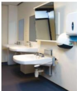
Fig. 6. Adjustable height wash hand basins and lever taps may be needed; hand-wash stations are installed at two height levels. [22]
