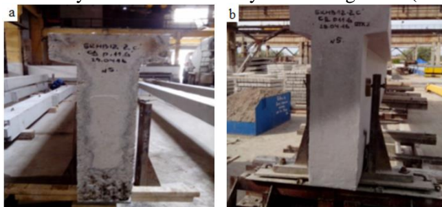
Fig. 1. Repaired precast crane by Nano cement a. Surface damage b. Crane after repair with Nano cement
