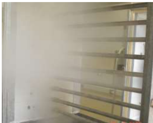
Fig. 3. Steam injection in the air duct
