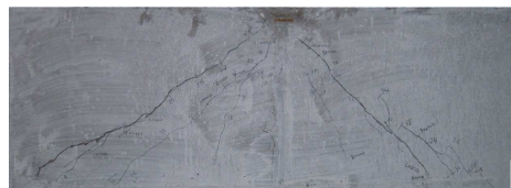
Pattern of cracks of beam B_6
