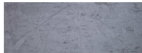
Pattern of cracks of beam B_{10}
