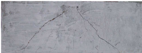
Pattern of cracks of beam B_3
