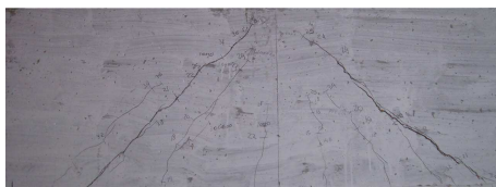
Pattern of cracks of beam B_7
