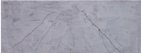
Pattern of cracks of beam B_1
