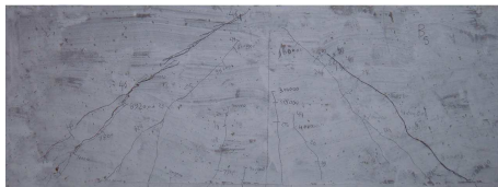
Pattern of cracks of beam B_5
