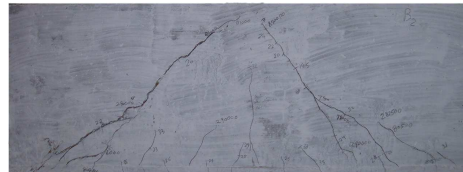
Pattern of cracks of beam B_2
