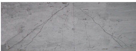
Pattern of cracks of beam B_9
