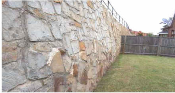
Photo 2. Severe Wall Distress.
