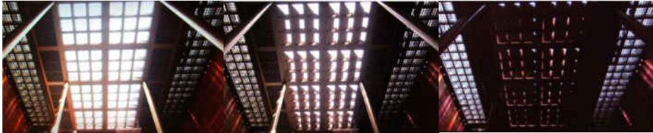
Fig. 10. A roof covering for an open-air plaza, Aldar Central Market, Abu Dhabi, UAE. [15]
