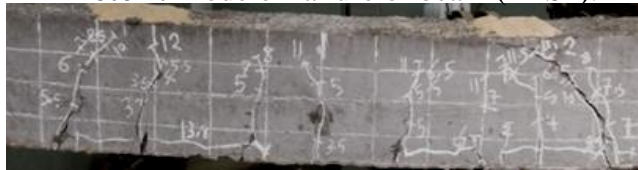
Photo 8. Mode of failure of beam (BFS3).
