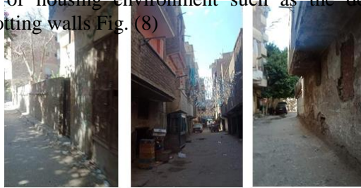
Fig. 8. Buildings deterioration and low quality.(By: researcher, 16-6-2019)
