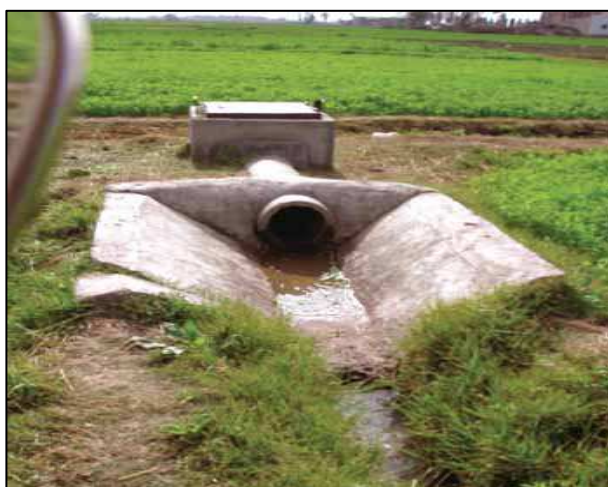
Photo (3) Buried pipeline Mesqa
