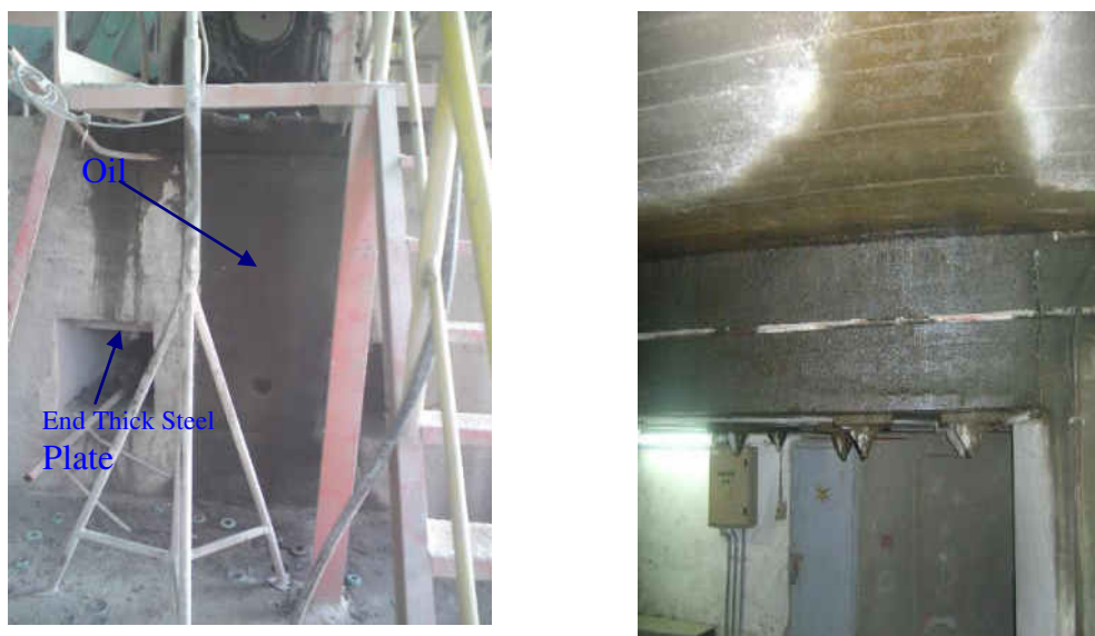
Fig. 6. Foundation of crusher contaminated by mineral oil
