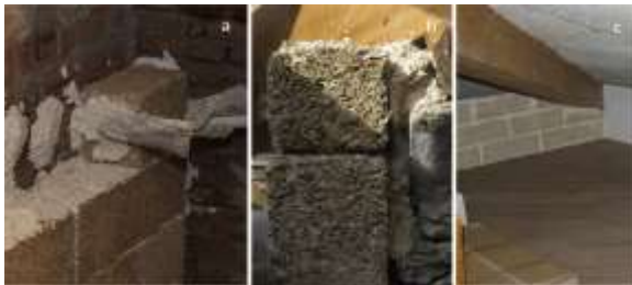
(Figure12) Details of non-load-bearing walls made of hemp-Crete blocks: (a) wall erection; (b) side view; (c) front view
