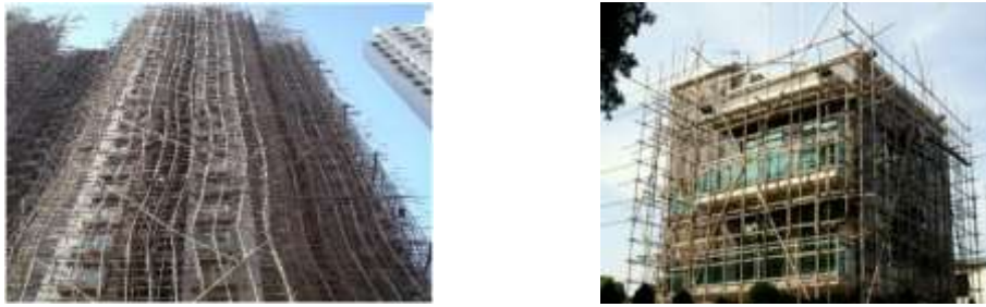
Figure 15 Bamboo scaffolding. Reproduced from Correal, J.F., 2016. Bamboo design and construction. In: Harries, K.A., Harma, B. (Eds.), Nonconventional and Vernacular Construction Materials.
