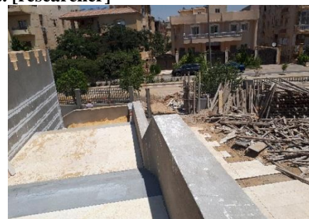
Figure 28: The finished external staircases with a width of 3.30 m to meet the code requirements. [researcher]
