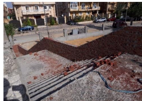
Figure 27: Adding a concrete wall staircase to comply with the total widths of the required stairs. [researcher]
