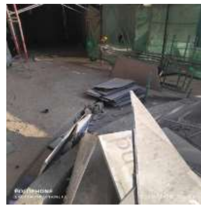
Figure9:Bad storage material
