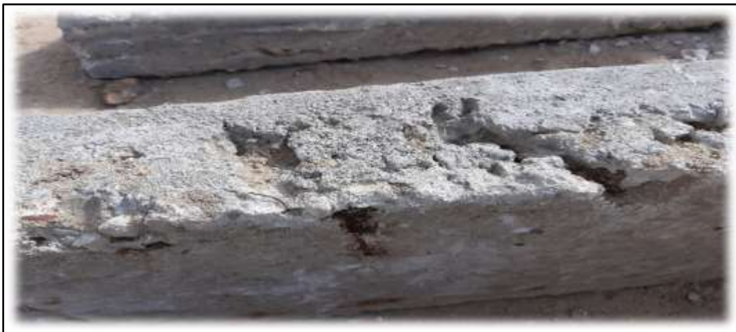
Figure 2. Beam B3 after it was exposed to offshore climate before being repaired.
