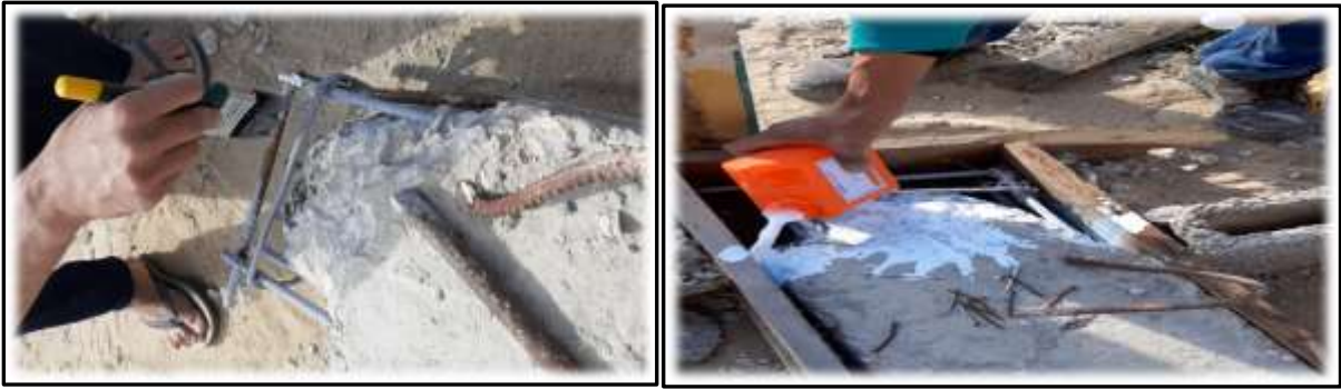
Figure 4. Beam B4 after being repaired with Sika zinc rich epoxy and adebond.
