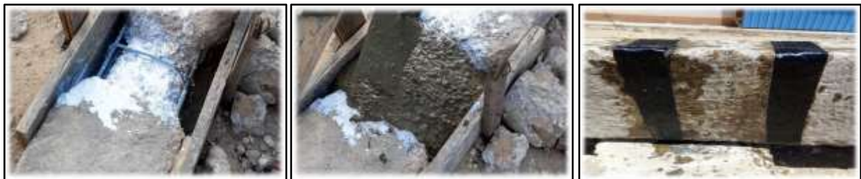
Figure 5. Beam B5 after being repaired with Sika zinc rich epoxy, adebond and CFRP.
