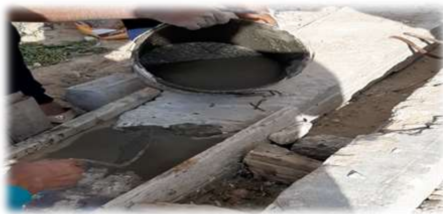
Figure 3. Beam B3 after being repaired with Sika zinc rich epoxy and Grout.
