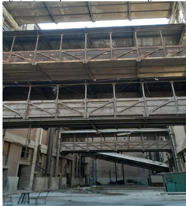
Source: The researchers Fig. (18g) view of Masr press roof overlooking western part.
