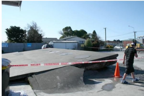
Fig. 1. Petrol tank uplift - Christchurch Earthquake [6].
