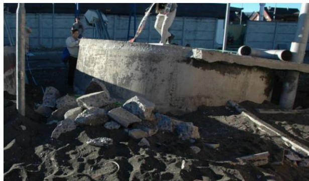
Fig. 3. Uplifted sewage tank - 2010 Chile Earthquake [8].
