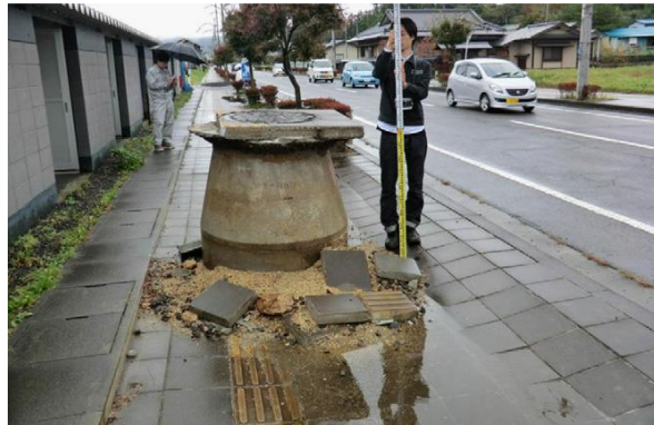
Fig. 2. Uplift of a manhole – Tohoku Earthquake [7].
