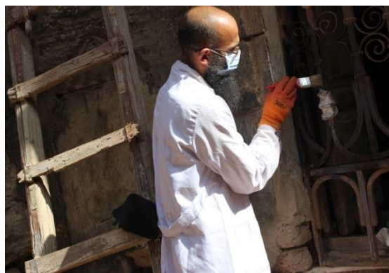
Fig. 9: iron window grille was coated by tannic acid dilutes in alcohol 3% by brush.
