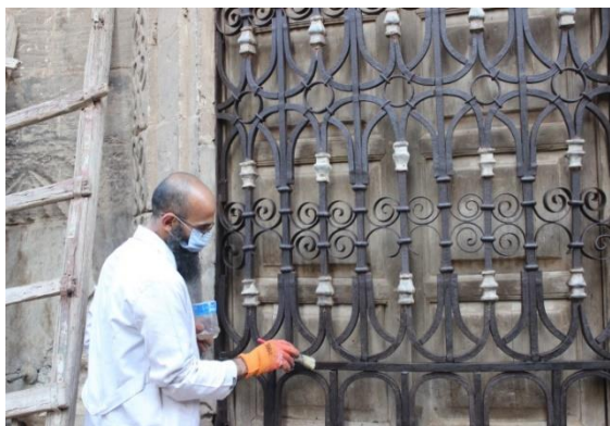
Fig. 11: The iron window grille was coated with polyamide 2% which applied in two layers by brush, from top to down and another layer from right to left
