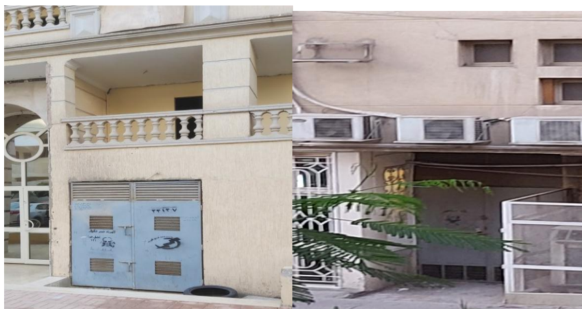
Fig (11): transformers placed inside residential buildings
