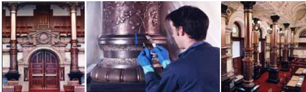
Figure 12. Bronze Columns at the Kansas State Capitol Senate Chamber, Metal Architectural Elements at the Kansas State Capitol Senate Chamber, Bronze Conservation Treatment. The Senate Chamber was a unique artistic work ornamented in 1885. The round windows, which feature faceted stained glass, were imported from France. The walls were decorated with various exotic materials from all over the world.
