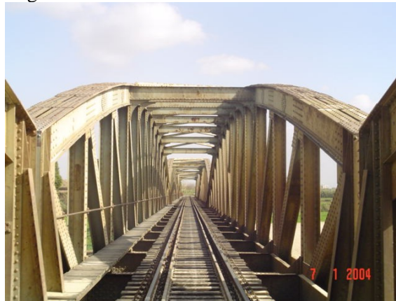
Figure 16. Qanater Bridge Condition before Strengthening Applications
