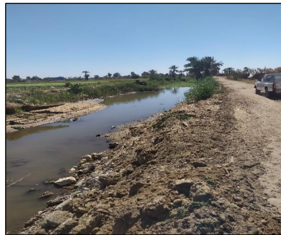
Photo (6): Failure of canal side slopes
